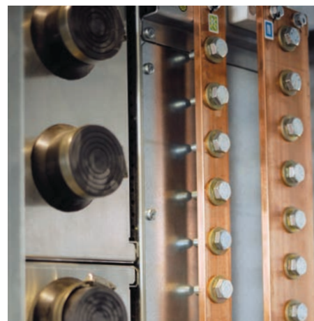
Maximum protection provided by segregation walls and partitions
